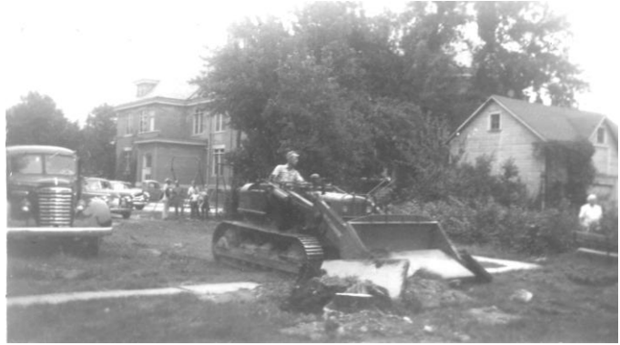
Site of former convent building on Kendall Street being cleared so the new brick convent could be built.
